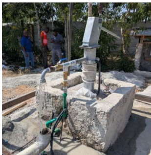
Operated by solar powered pump
