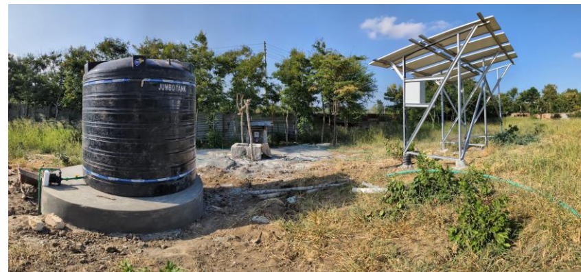
Overview of hybrid system (water tank, solar panels, piping)
